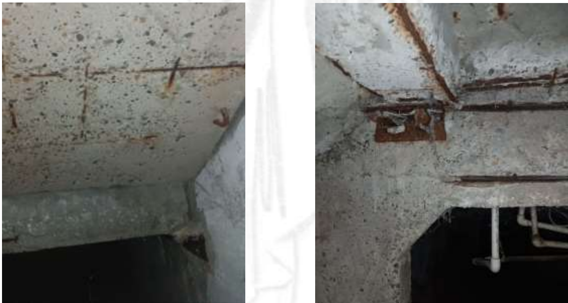
Figure 1. The effect of moisture (chloride ions) in the basement of a building on reinforced concrete structures.
